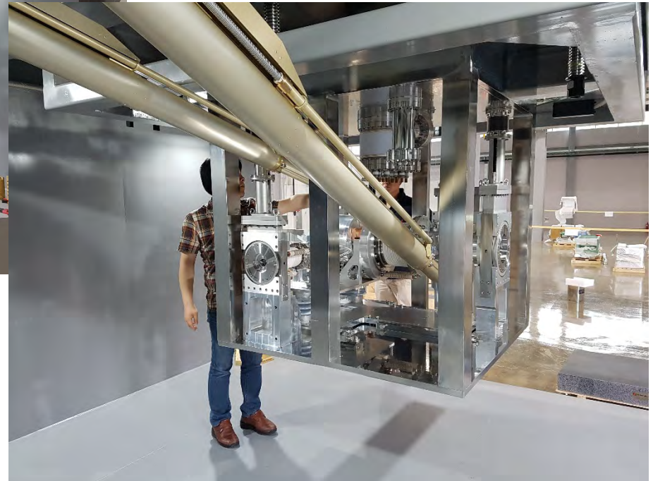
* Inside Hot-cell & Manipulator
